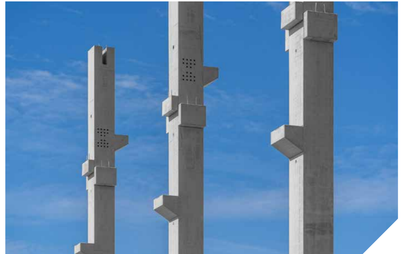
Siemens, Budapest Year of handover: 2023. Delivered products: complete prefabricated structure Floor area: 17.000 m 2 Produced quantity: 3.660 m 3
