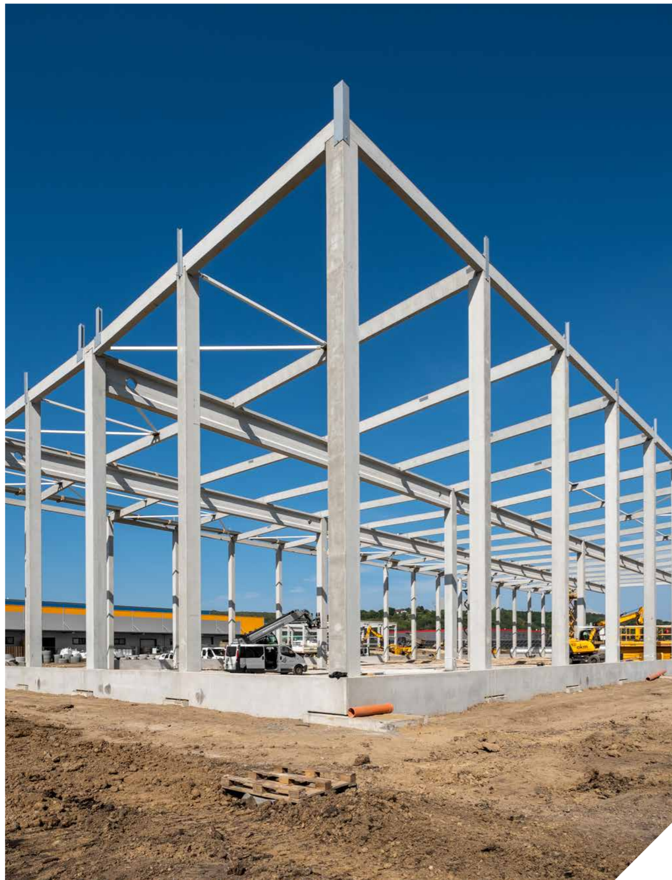
Ongropack, Szirmabesenyő Year of handover: 2024. Delivered products: complete prefabricated structure Floor area: 4.389 m 2 Produced quantity: 564 m 3
