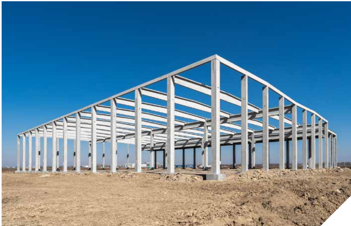
SEMCORP lithium-ion battery factory, Debrecen Year of handover: 2022. Delivered products: complete prefabricated structure Floor area: 48.000 m 2 Produced quantity: 5.900 m 3
